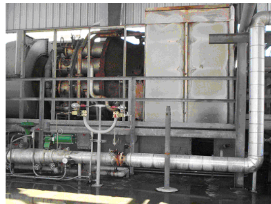
Figure 1: IR image of the combustor section of GE Frame 5 gas turbine and the corresponding photo.
